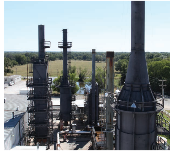
Burner test facility houses seven test furnaces
